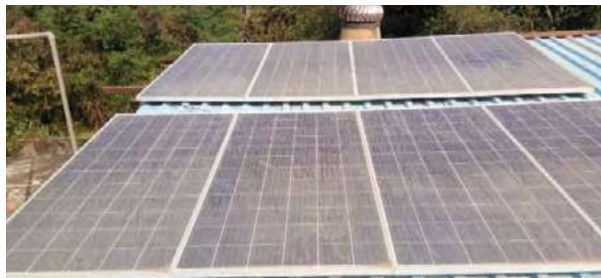
Solar Energy Setup
