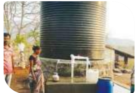
Water tank installed at Piwali village
