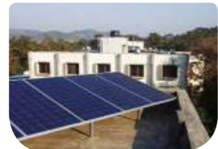
Solar Energy Setup in a School in Vasind, Maharashtra
